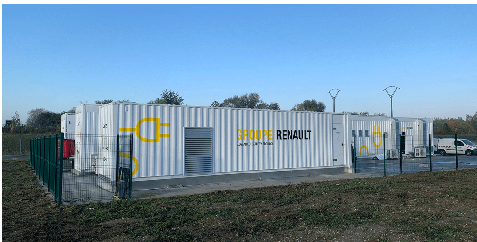
Figure 6-13. Batteries from Renault EVs are reused for stationary purposes. 203
