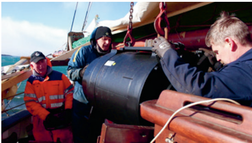
Figure 4. Installation of the permanent magnet motor into Opal.
