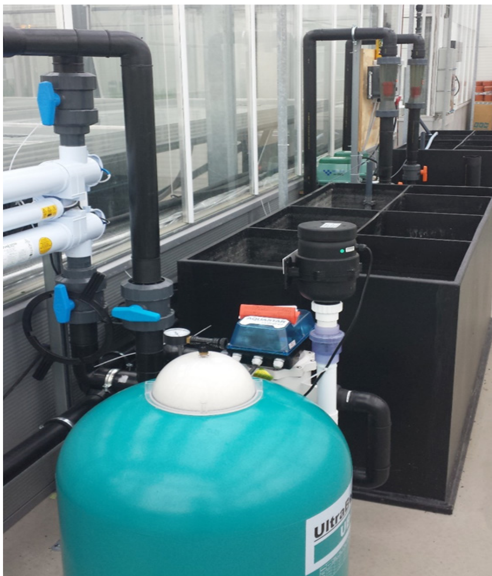
Figure 2.3-3: Bio-filter, UV-lighting, sedimentation tanks and airblower. Photo: Paul Rye Kledal, IGFF.
